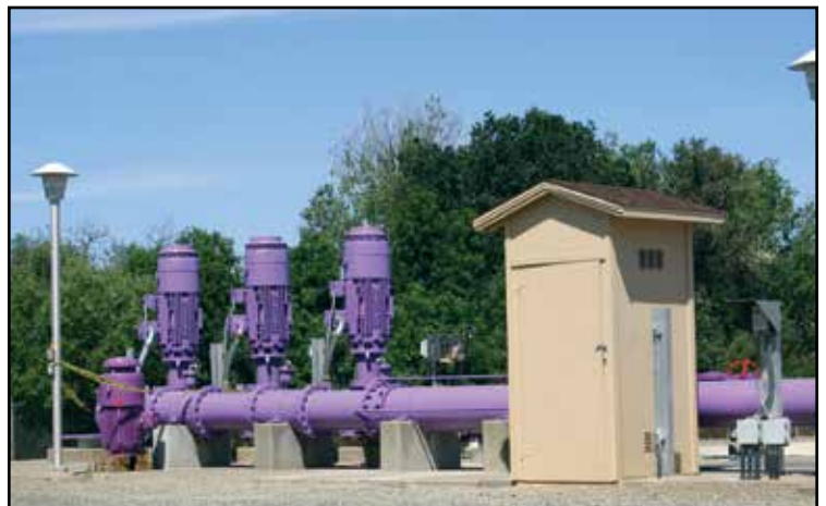
Recycled water is produced at EID's El Dorado Hills (pictured) and Deer Creek wastewater treatment plants. Pipes that convey recycled water are colored purple, from the treatment plant all the way to the recycled water users' landscapes.
